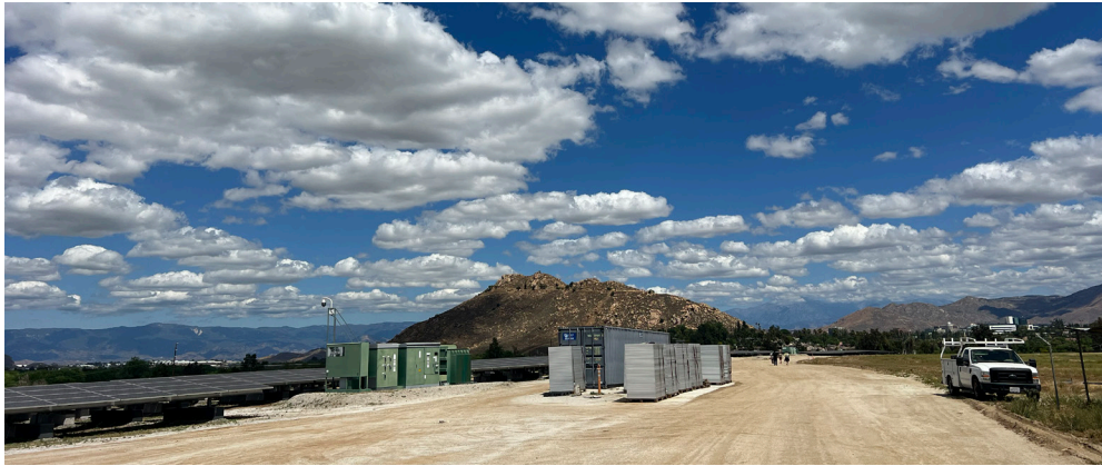
2. Maintenance truck, solar farm equipment.
