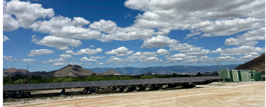
5. Solar panels and noisy transformer.
