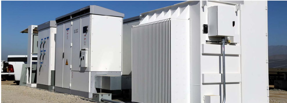
INVERTER CLOSE UP
