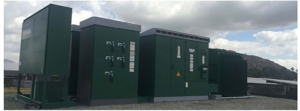
INVERTER CLOSE UP
