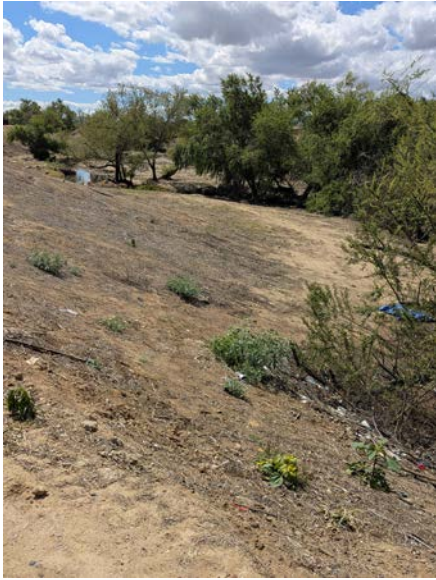
1. Eastern slope down to creek, debris
