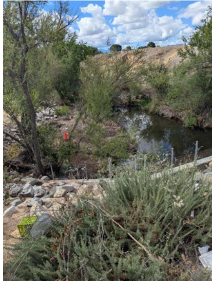
2. Riprap and trash in Hole Lake
