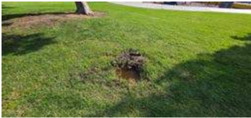
Problem with the Pipes
